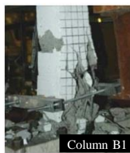
Pic.1 Damage State
