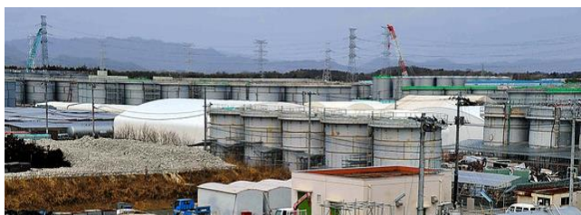
Fig1. Tank group in the nuclear power plant
