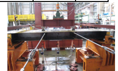
Photo1 Reinforcement prevented for Lateral buckling
