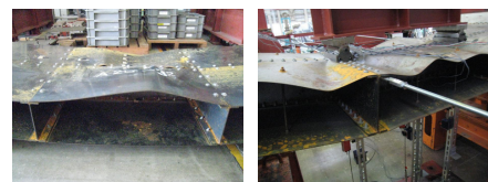
Photo2 Rib and thin steel panel buckling states
