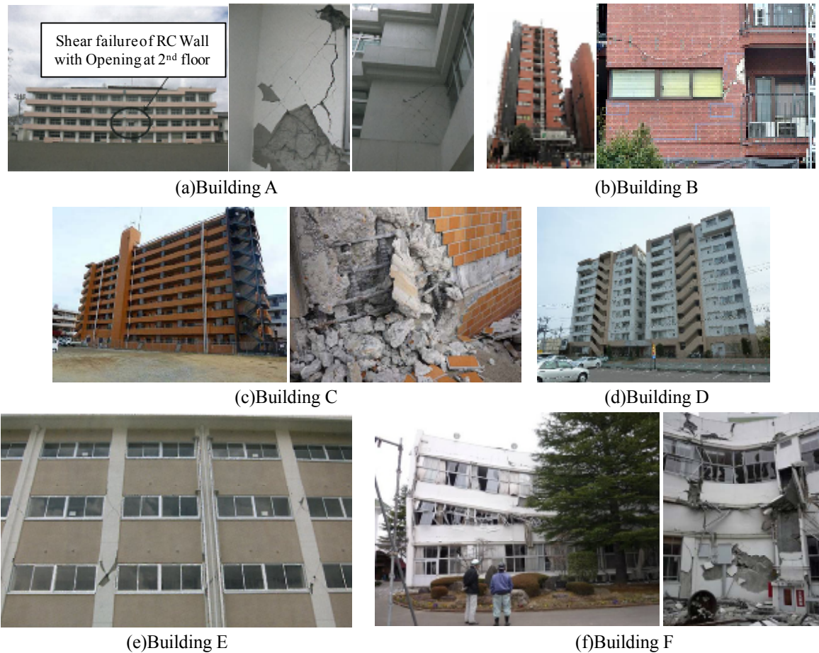
Figure 1 Damage Condition of Target Buildings
