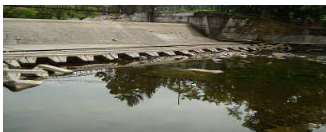
Photo 1. Local scour downstream of the weir at Power generation
