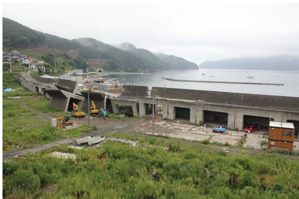
Fig.6 Broken tide embankments (Toni-cho, Kamaishi City)
