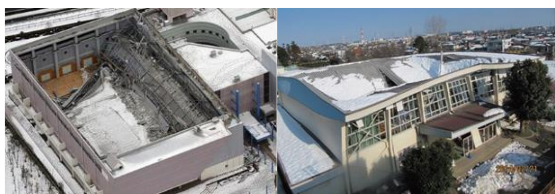
Figure 1 Heavy snow damage
