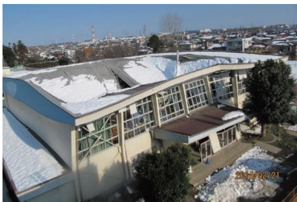
Figure1. Collapsed gymnasium roof [2]
