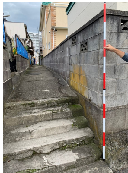
Figure4. A narrow passage in a residential area where there is a risk of falling objects
