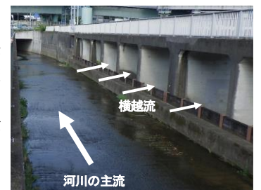
Photograph.1 Example of side weir (Bikuni-Bashi flood control reservoir at Shirako River in Tokyo, Japan)
